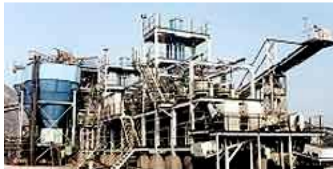
Industrial coal dust installations
